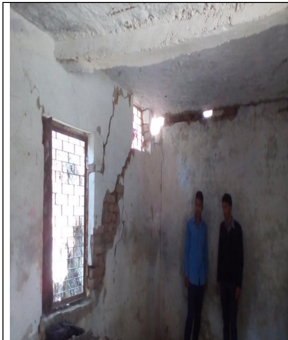
Wide cracks in walls and deflected beam
