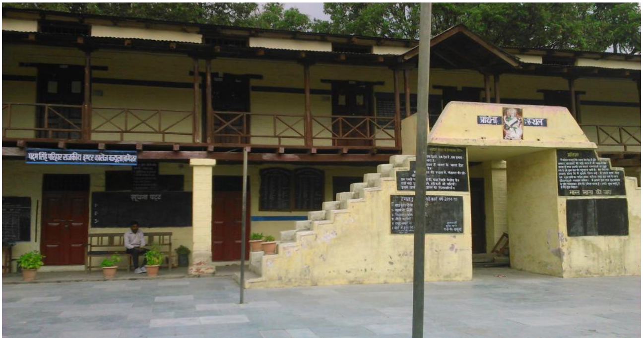
Irregularity in main Building.
