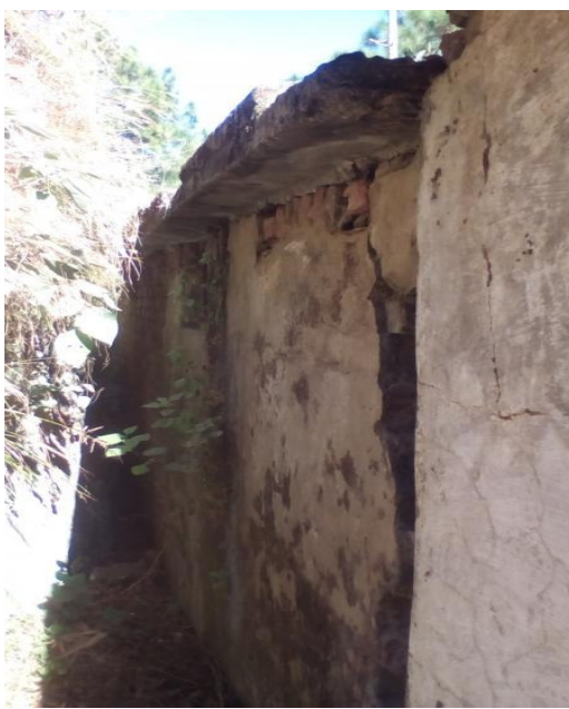
Backside wall is damaged
