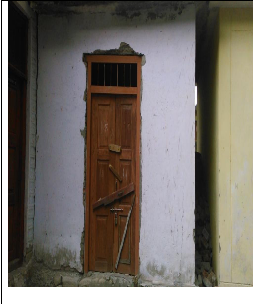
Lintel Band not provided
