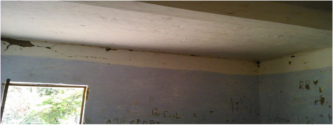
Cracks below the slab
