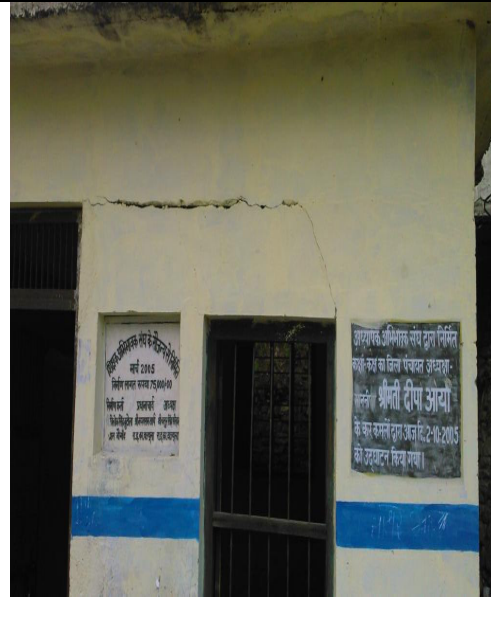
Major Crack above window
