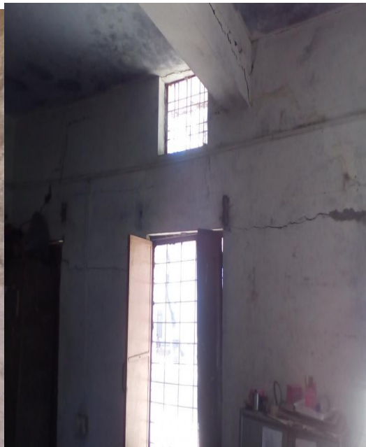
Major cracks in wall and beam
