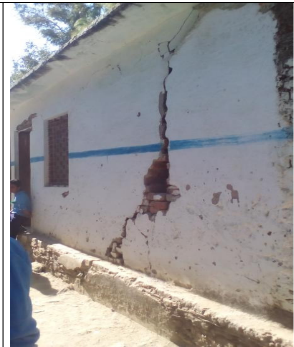
Shear cracks in beam
